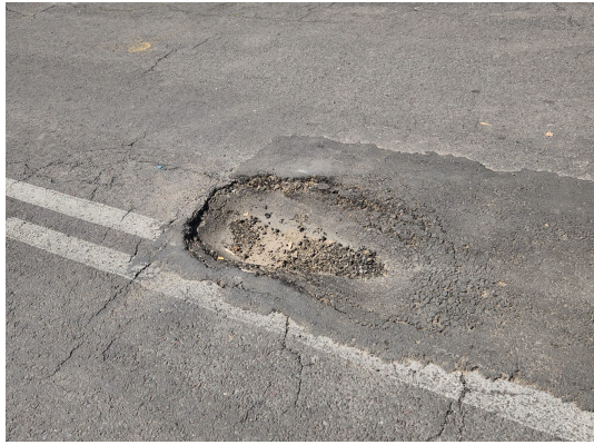
(a) A road with potholes.
