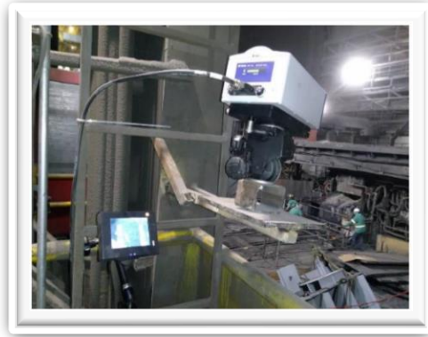
Fig. 6.8 Laser emitter installed in the steel shop
