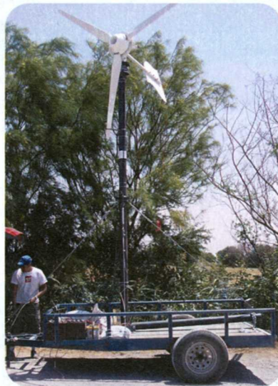
Figura 4.15: Turbina instalada y pivoteada.
