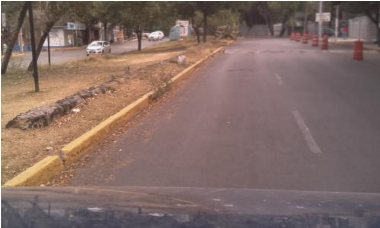
Figure C-12. OBU photograph before a pothole and a speed bump.
