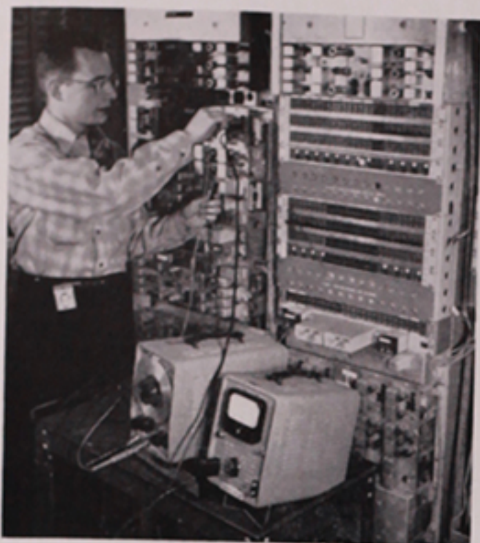
Fig. 5—G. W. Carter performing a transmission test on Laboratories Type-ON terminal equipment.
